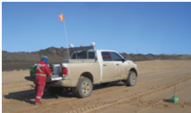
A Norwest construction monitoring technologist collects and records compaction and other construction data in the field.
